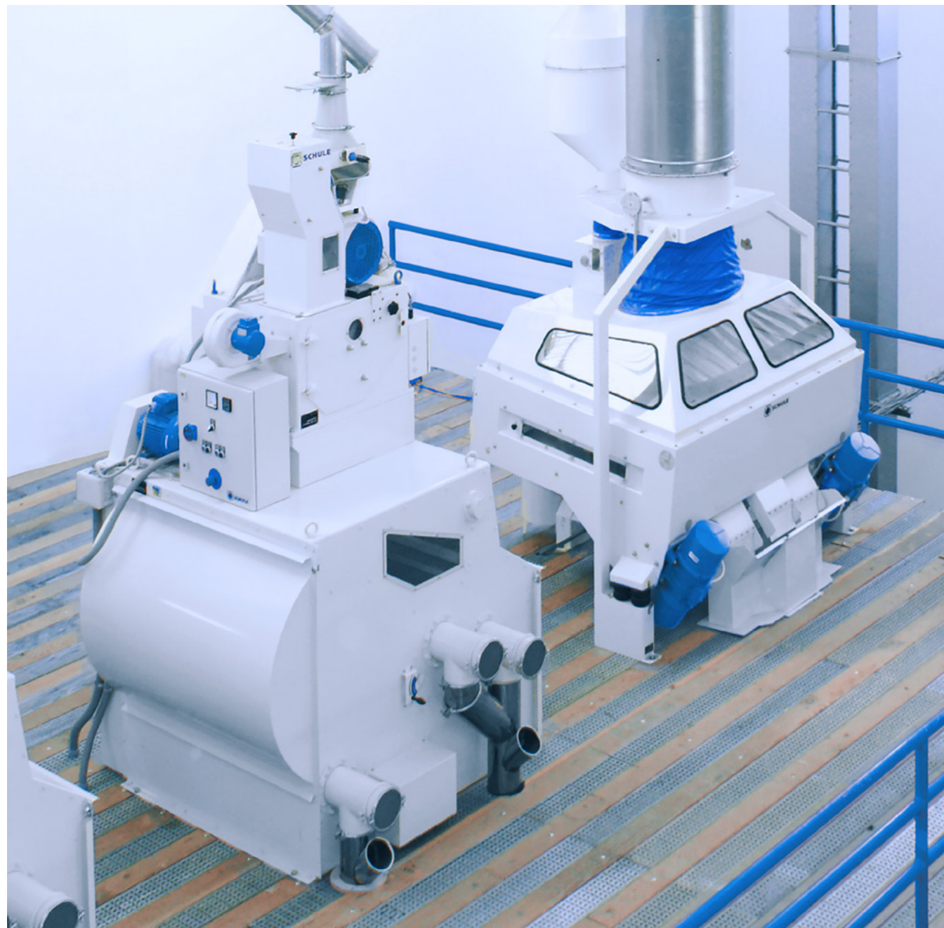
↑ View into a SCHULE rice plant
